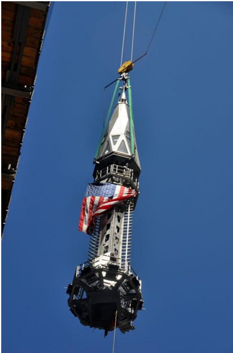
The top of the One World Trade Center spire as it is lifted off the ground.
