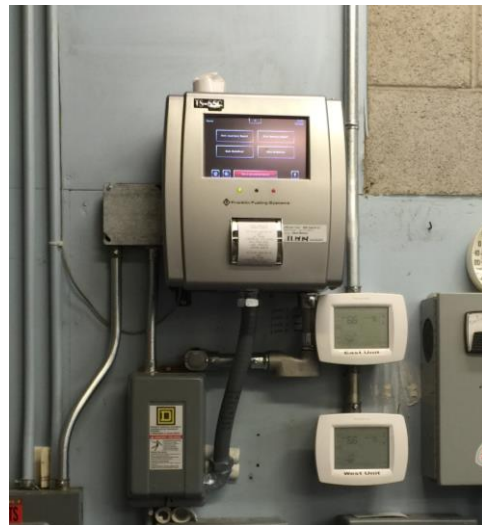
Fig 3 Fuel Monitoring System
