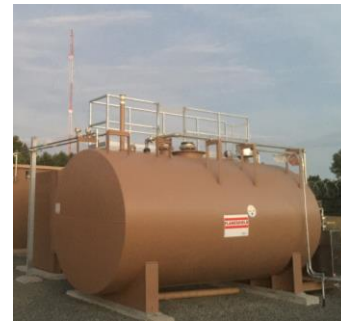
Fig 2 6,000 Gallon, Double-Walled Fuel Tank
